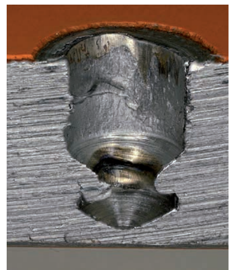
Steel base material after 10 years of exposure to sea water and pull-out of the X-BT fastener. The hole appears clean and no evidence of corrosion is visible.
